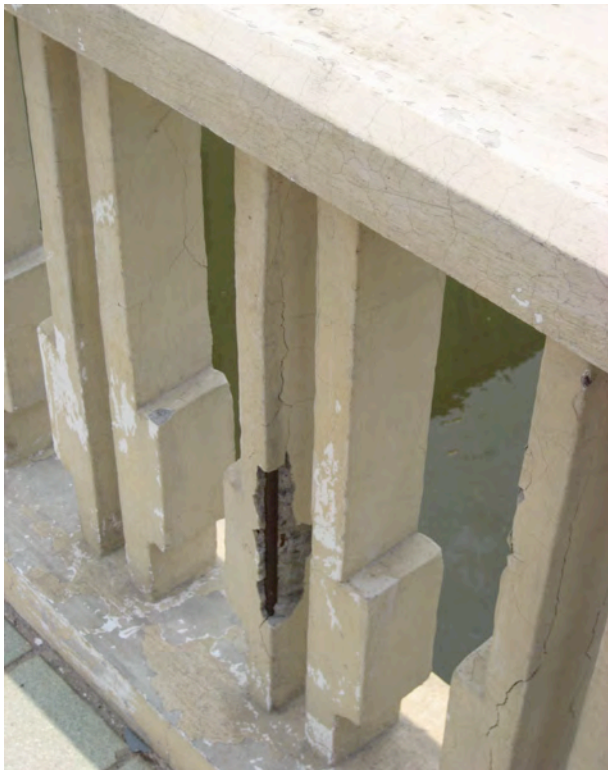
Photograph 23: Cracks in the newness of Anting architecture (own photo)
