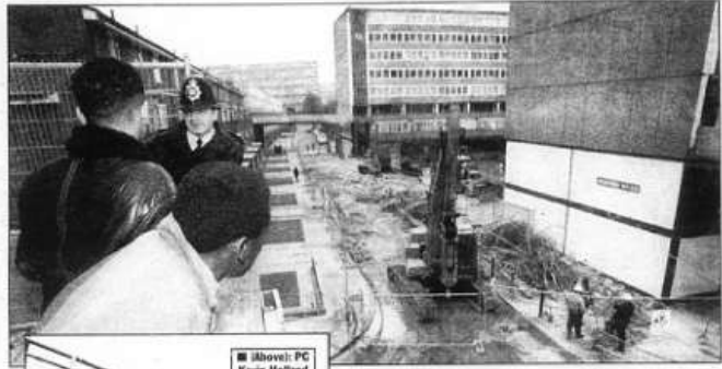
■ Above: PC Kevin Holland joins local youngsters as the Aylesbury Estate's walkways are demolished
