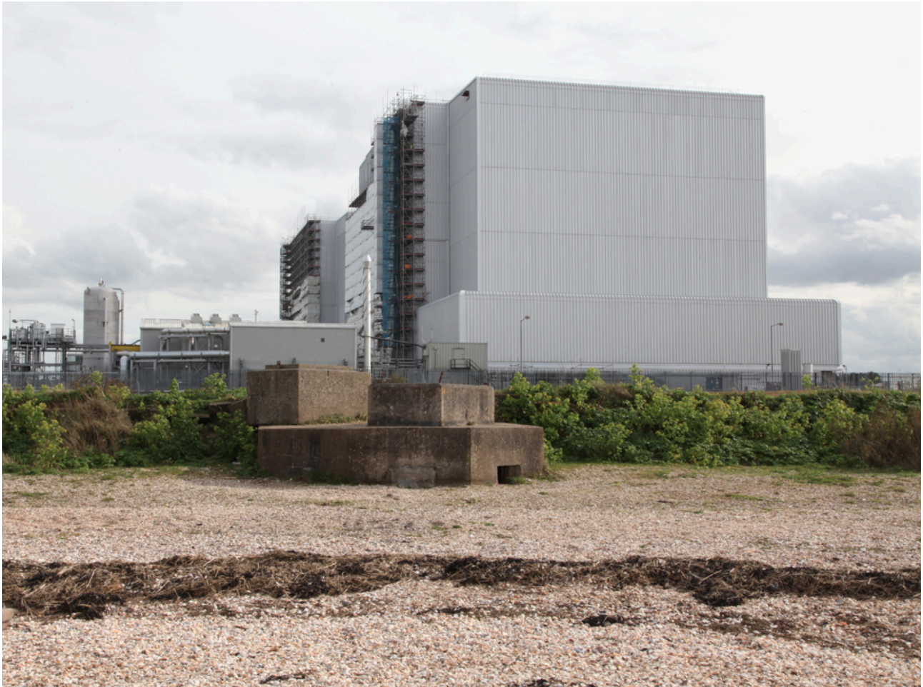
Figure 5: Bradwell A reactor buildings with the aluminium 'weather envelope' in construction to encase them. Photograph courtesy the author.
