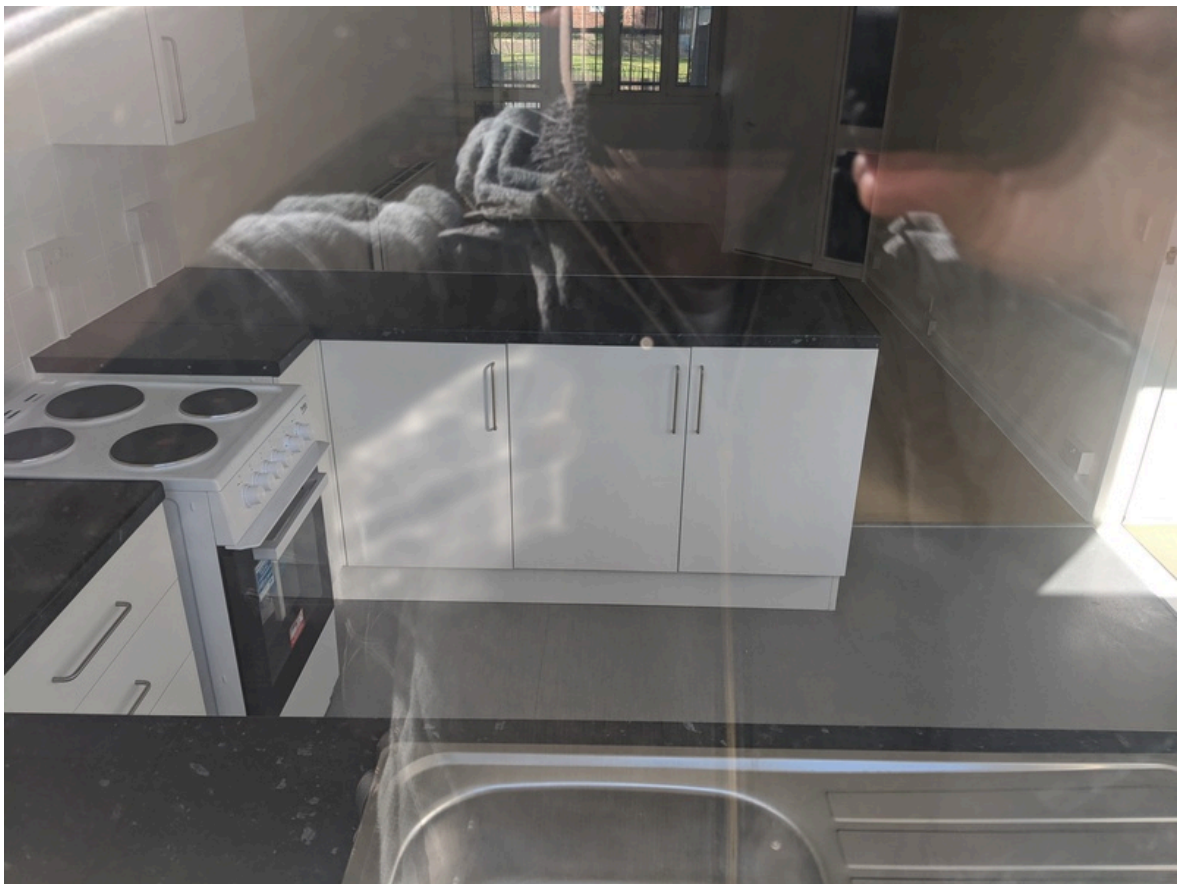
Figure 123. Refurbished flat on Cressingham once covered in black mould.
