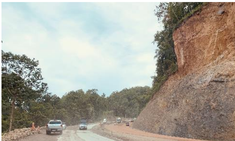
Figure 18: Road under construction. The road from Tak city to Mae Sot, through the mountains was under construction for much of my fieldwork.
