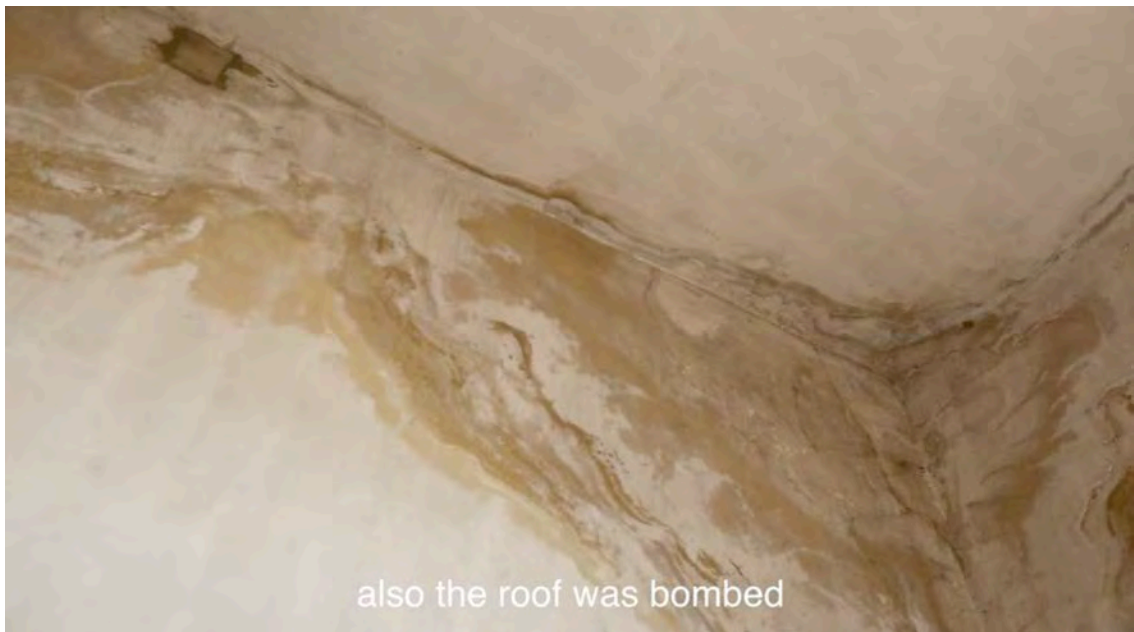
Figure 54: Soubhi Antonios points to the damage to his house in the 1941 Allied bombardment—there is still a material trace where the new cement hasn't fixed, allowing water to leak through. As featured in my film Under Multiple Suns . Masaar Al Chouf, Lebanon, 2017.
