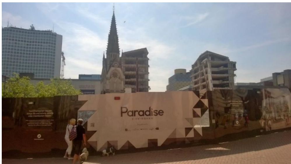
Figure 5.4: View of the demolished Central Library with LoB visible between the ruins.
