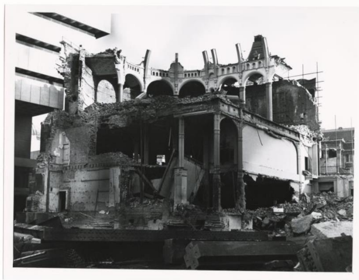
Figure 4.18: Partially demolished old Birmingham Central Library (1882) adjacent to the new one (1973) (Images: Birmingham Archives and Heritage, 2016)
