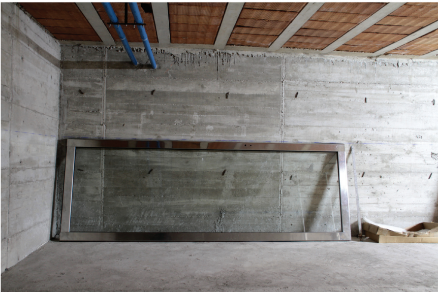
FIG. 6.11 Broken door in the basement of the Barcelona Pavilion (photo: Andrés Jaque, 2012)
