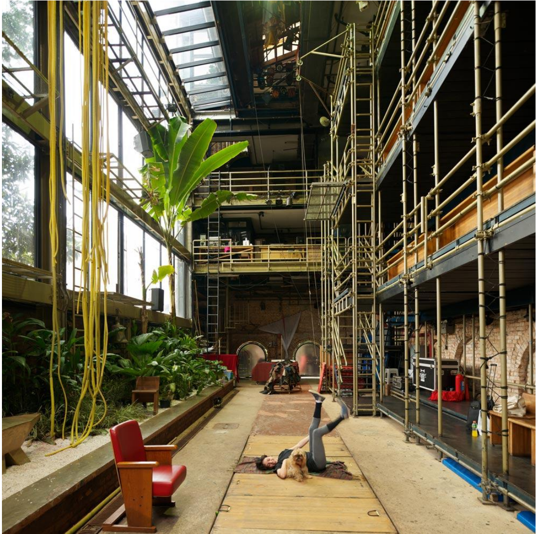
8. Teatro Oficina Uzyna Uzona Building conceived by Lina Bo Bardi (*picture from an architectural magazine, not from a performance) São Paulo
