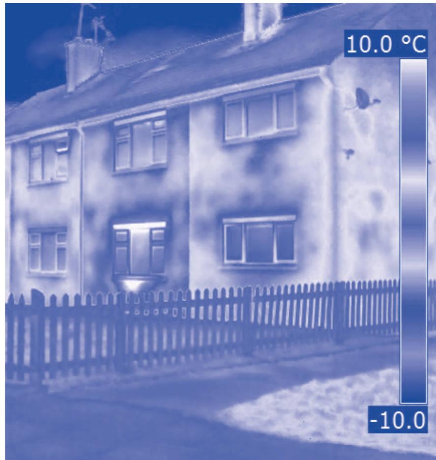
Thermal image of brick cavity wall dwelling with retrofitted insulation; note areas of potential heat loss
